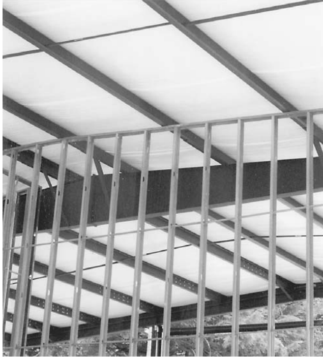
FIGURE 11.11 All-too-common practice: The interior partition is attached directly to roof purlins without any provision for accommodating vertical deflections. The partition will be forced to behave as a load-bearing wall and could fail when vertical roof load is applied.
